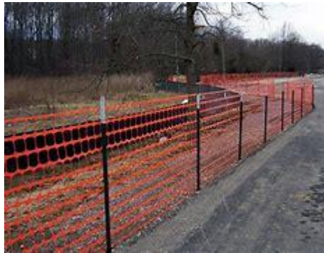
Mesh fencing is not sufficient to protect a pedestrian from falling into a trench or holes
